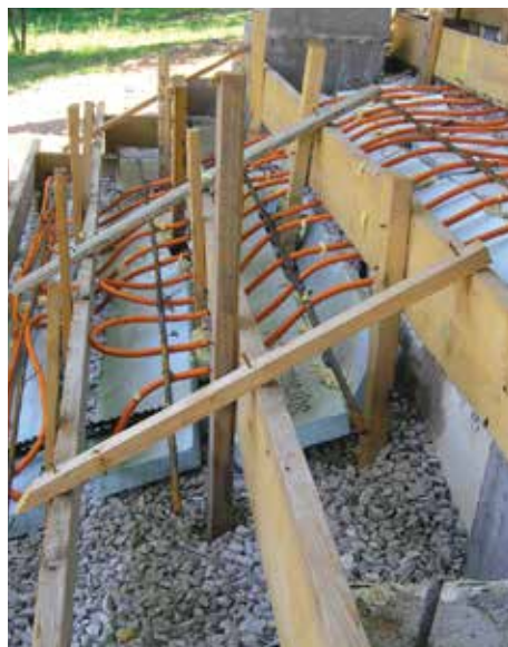
RadiantPEX-AL bends to conform to the shape of outdoor steps for snow melting.
