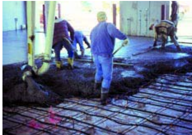
Onix being installed in multiple truck servicing bays.
